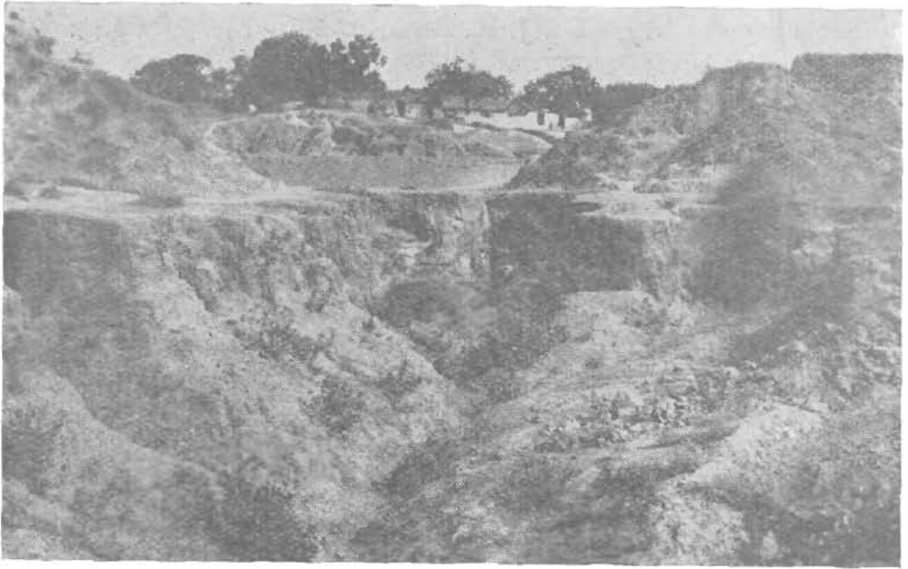
A view showing the gully behind the Post Office at village Bagchini and the diversion bund constructed to protect the further encroachment of the gully in the village.
