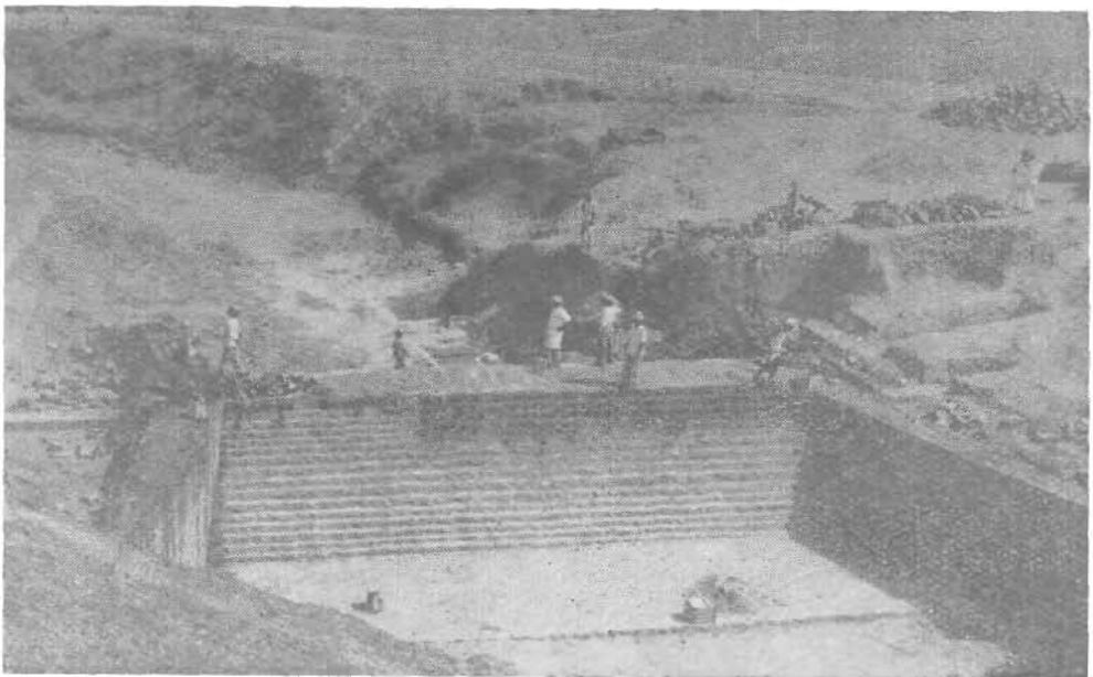
Masonry plug under construction in the Ravine Reclamation Scheme at village Bagchini, District Morena,
