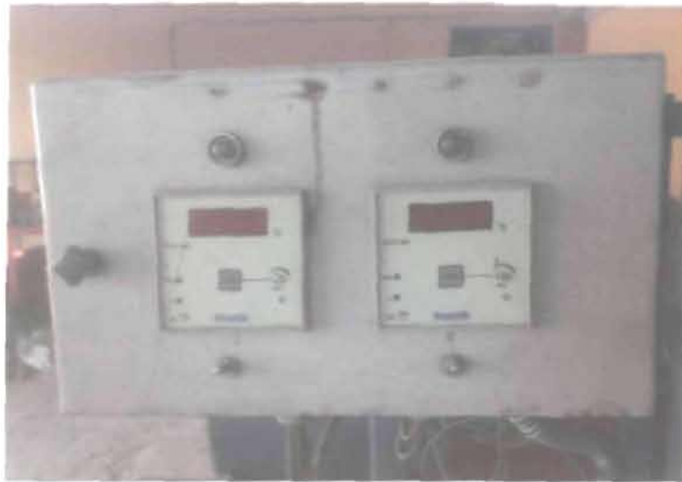
Plate 4.5 Temperature control panel for Mica band heaters of preheater
