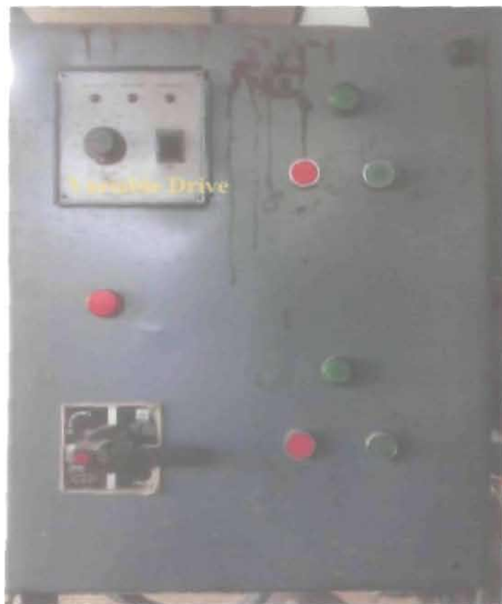
Plate 4.6 Briquetting machine control panel with variable drive for Preheater
