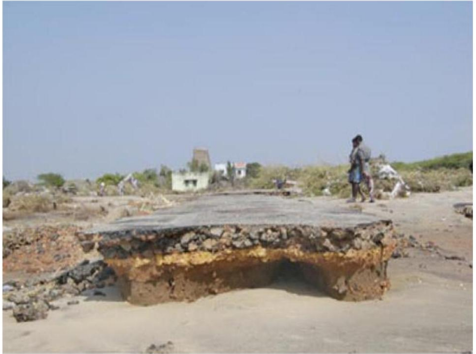
Plate 14. Link road eroded by Tsunami
