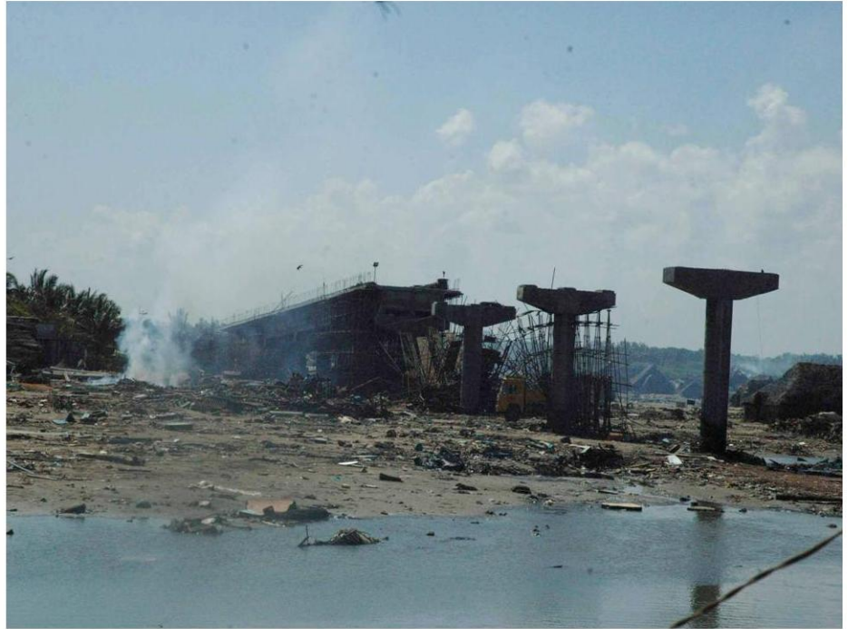
Plate 16. Bridge damaged by Tsunami waves
