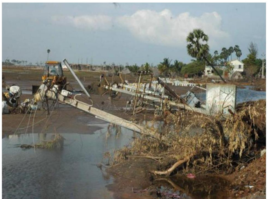
Plate 21. Electric post damaged by Tsunami
