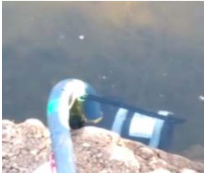
Fig. 3.3 (b):- DC Submersible Pump installed in the water source
