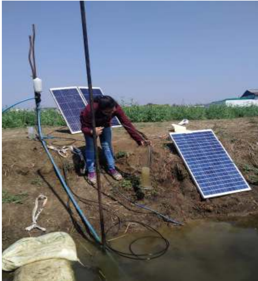
Fig 4.2:- Developed low head solar powered pumping system
