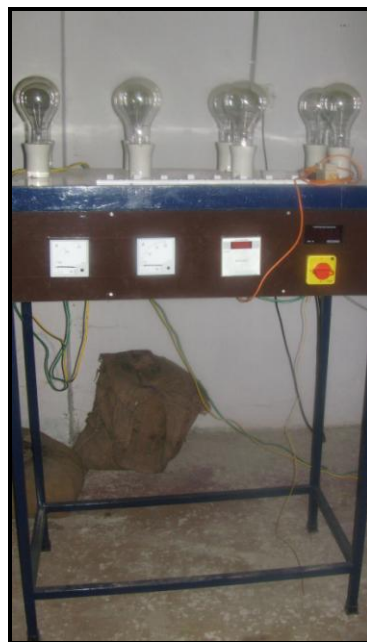
Fig. 4.11 Instrument control panel
