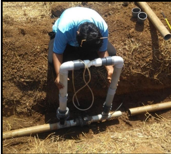
Plate 4.1 Installation of the developed device for fertigation in the field
