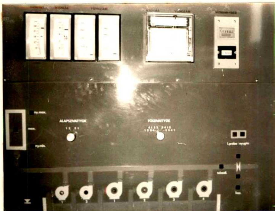
Fig.3.9 Instrumentation panel for indicating various parameters
