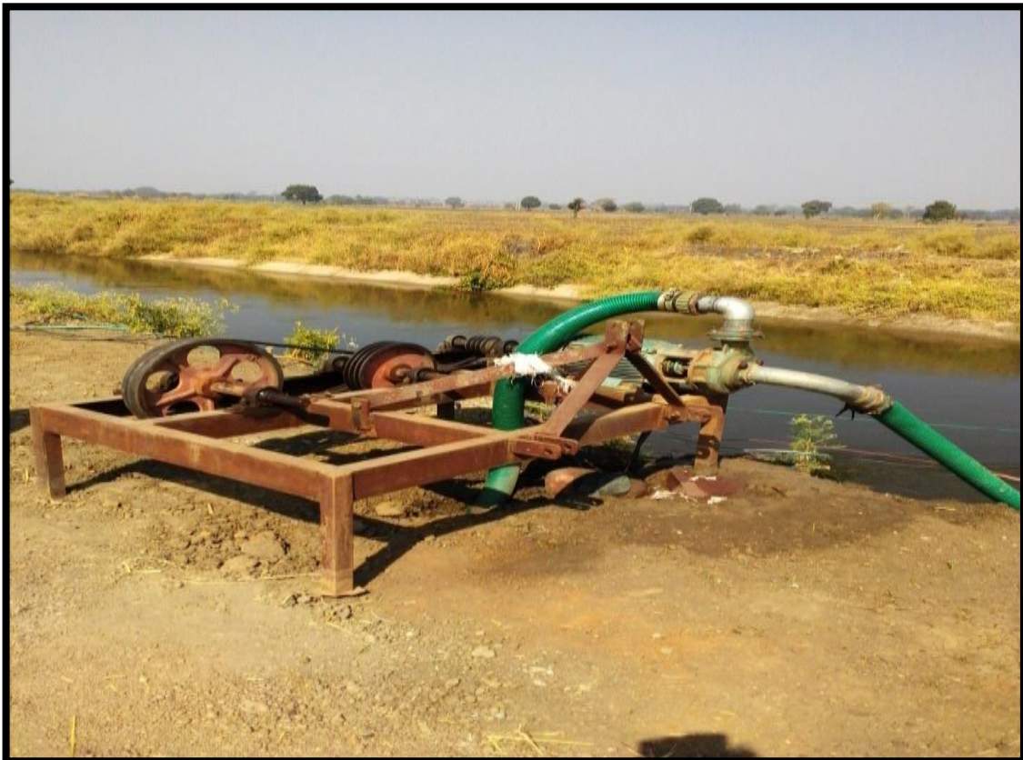
Plate 3.1 Lift of Water in Right Bank Canal Command
