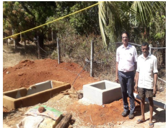
Plate 5: Fixed type biogas plant
