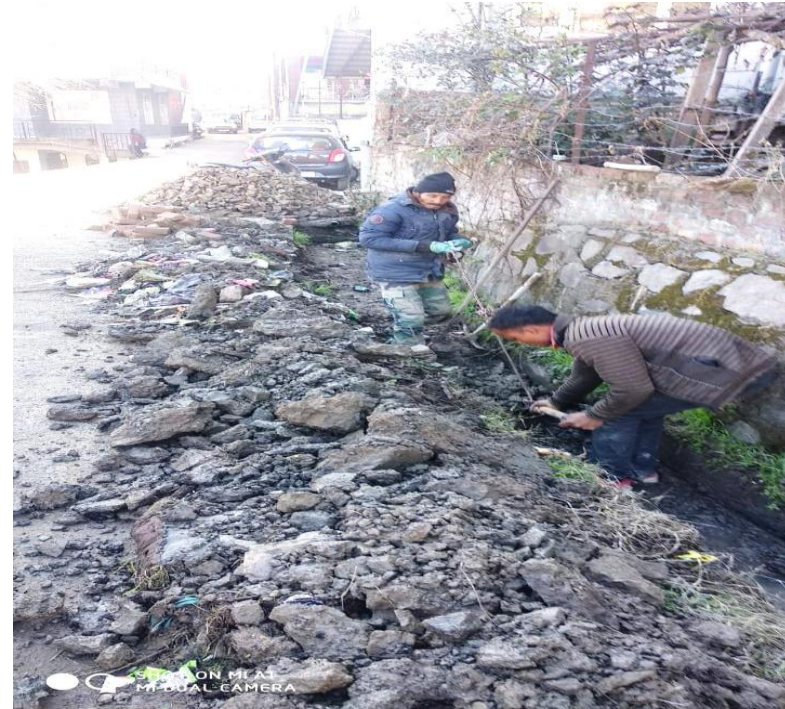
Fig 4.10 Drain pipe being installed in panchayat Saproon, Solan district under sanitation activities carried out by panchayat
