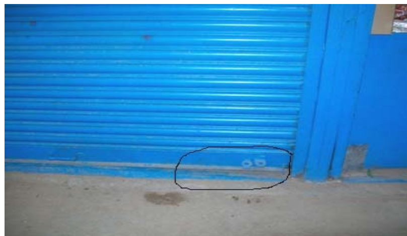
Plate 4.9 : Improper fitting of store
