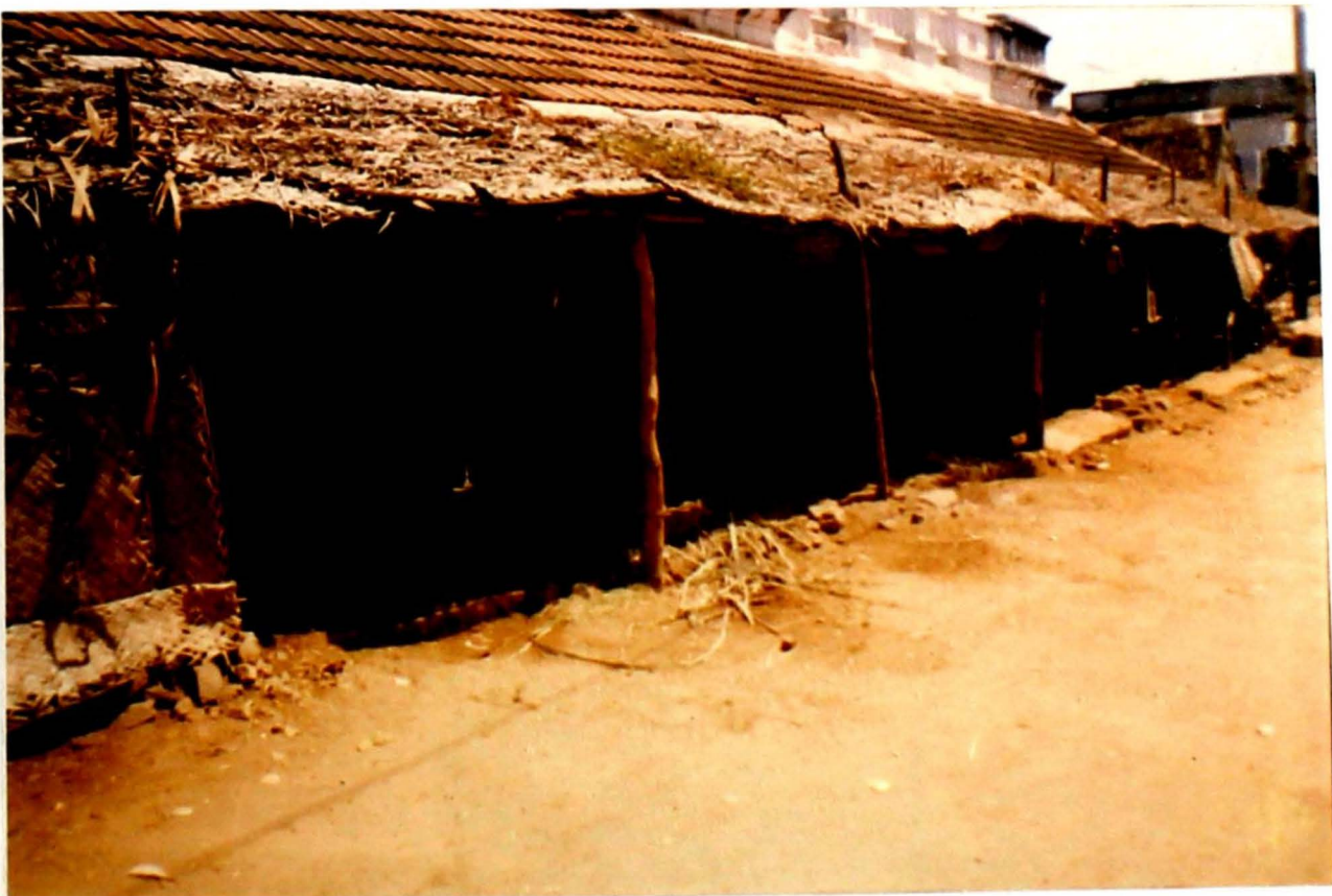
Plate No. 2. A view of front portion of house partly being used as cattle shed
