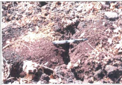
← Wide cracks in Masala soils
