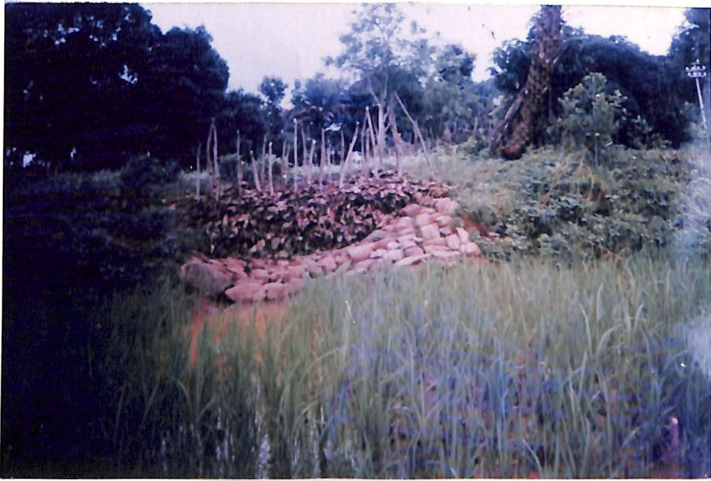
Plate No. 6 Combined structure of loose rock and brushwood on the field bund
