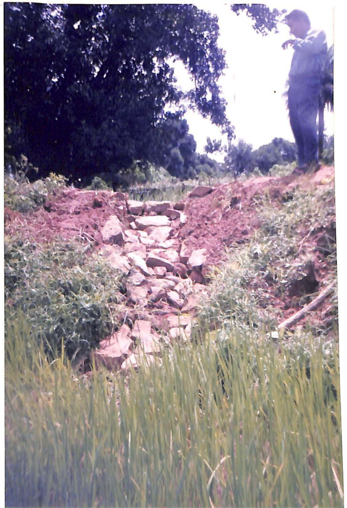
Plate No. 5 Loose rock structure on field bund
