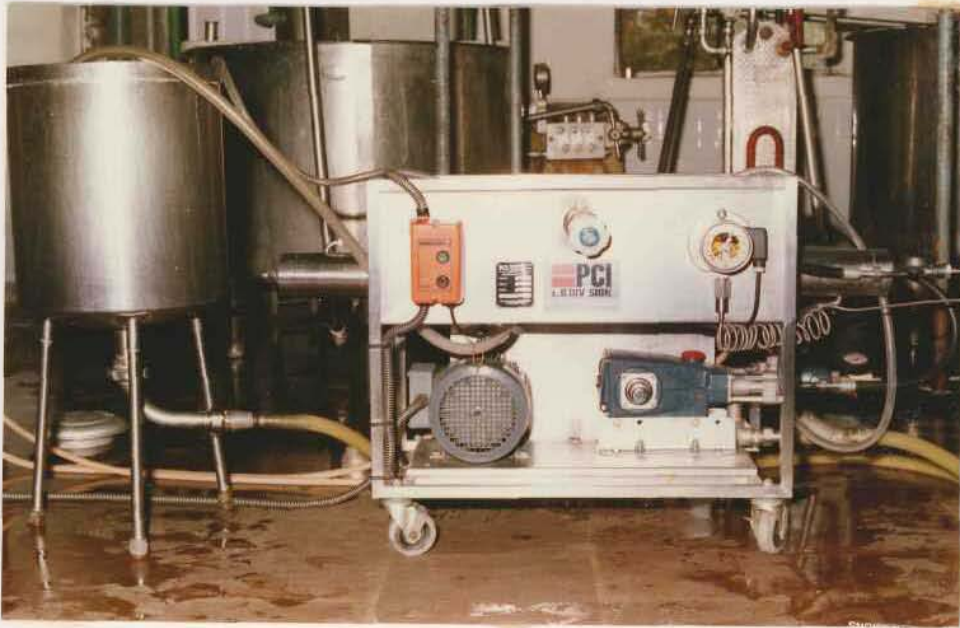
PHOTO PLATE 1 : REVERSE OSMOSIS PLANT
