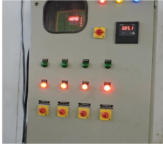
Picture 1: Temperature-Humidity Control Panel
