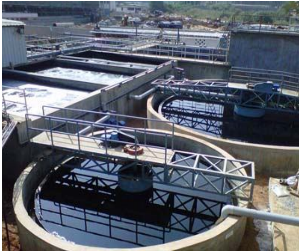
Fig.14: Effluent Treatment Plant
