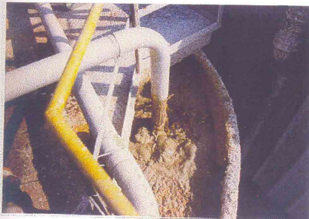
Plate 2 Thickner slurry pump site
