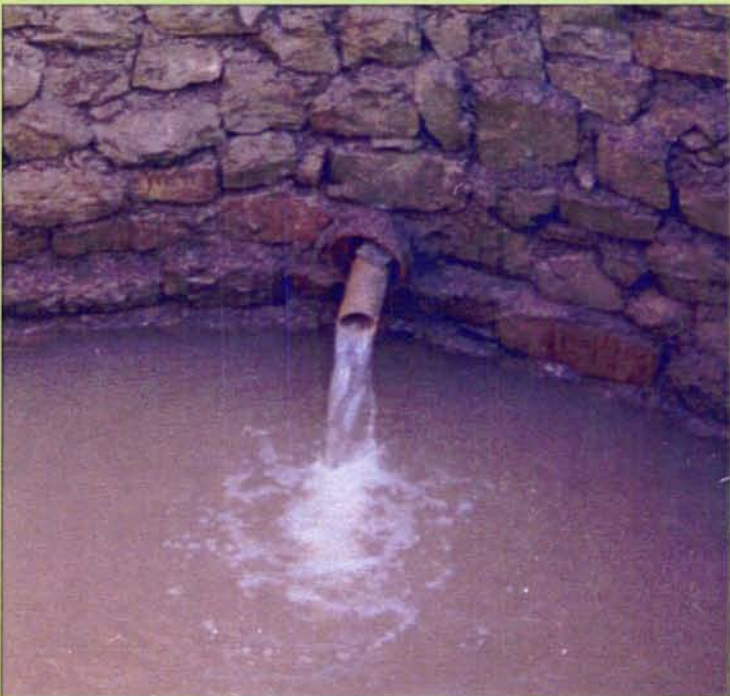
C) Collector drain discharging drain water in sump well on research field
