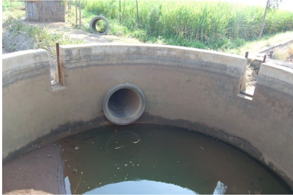
Plate 3. Water supply from intake well to reservoir
