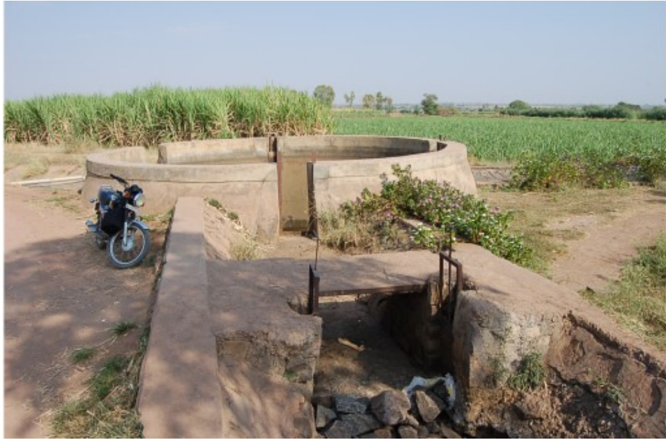
Plate 1. Reservoir to store water from intake well
