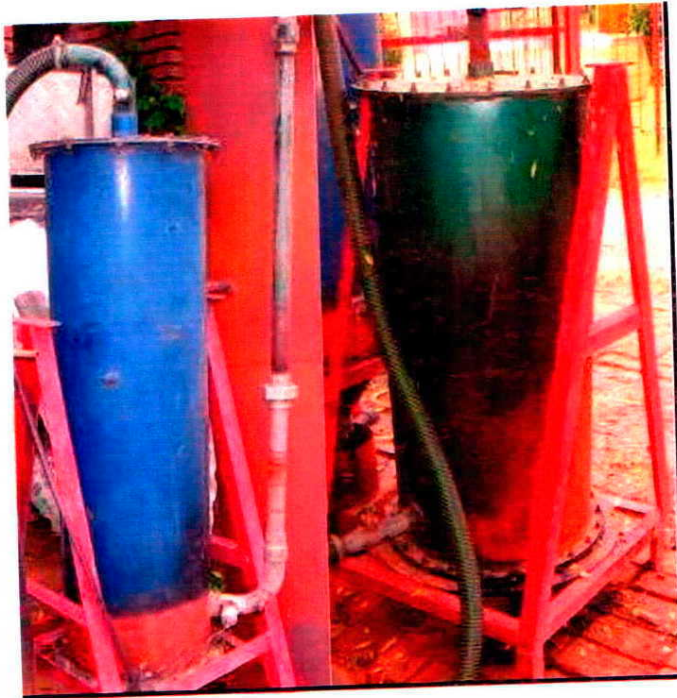
Fig. 3.7 Gas cleaning system
