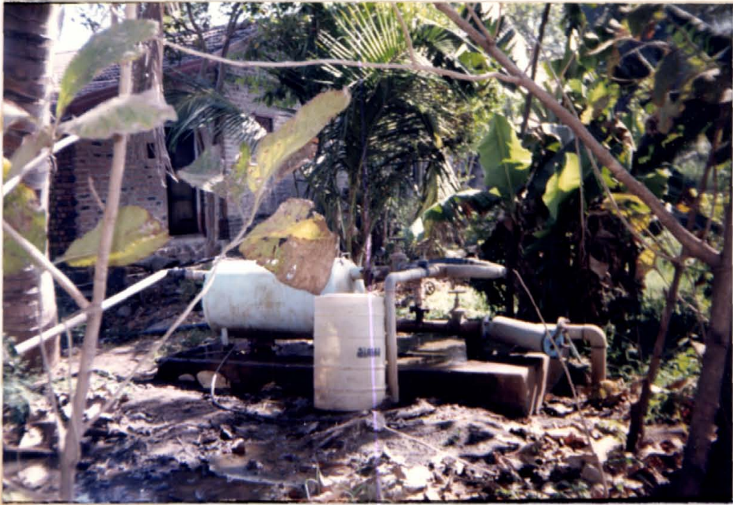
Plate-3 : Biwall drip irrigation unit
