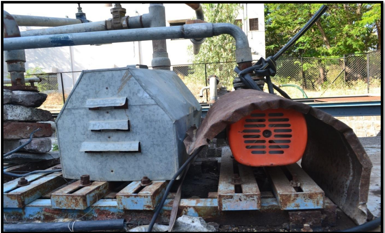
Plate 3.4 Pump set used for irrigation
