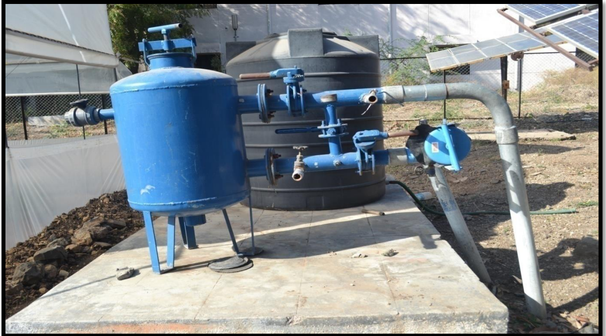
Plate 3.5 Filter unit assembly of the drip irrigation system
