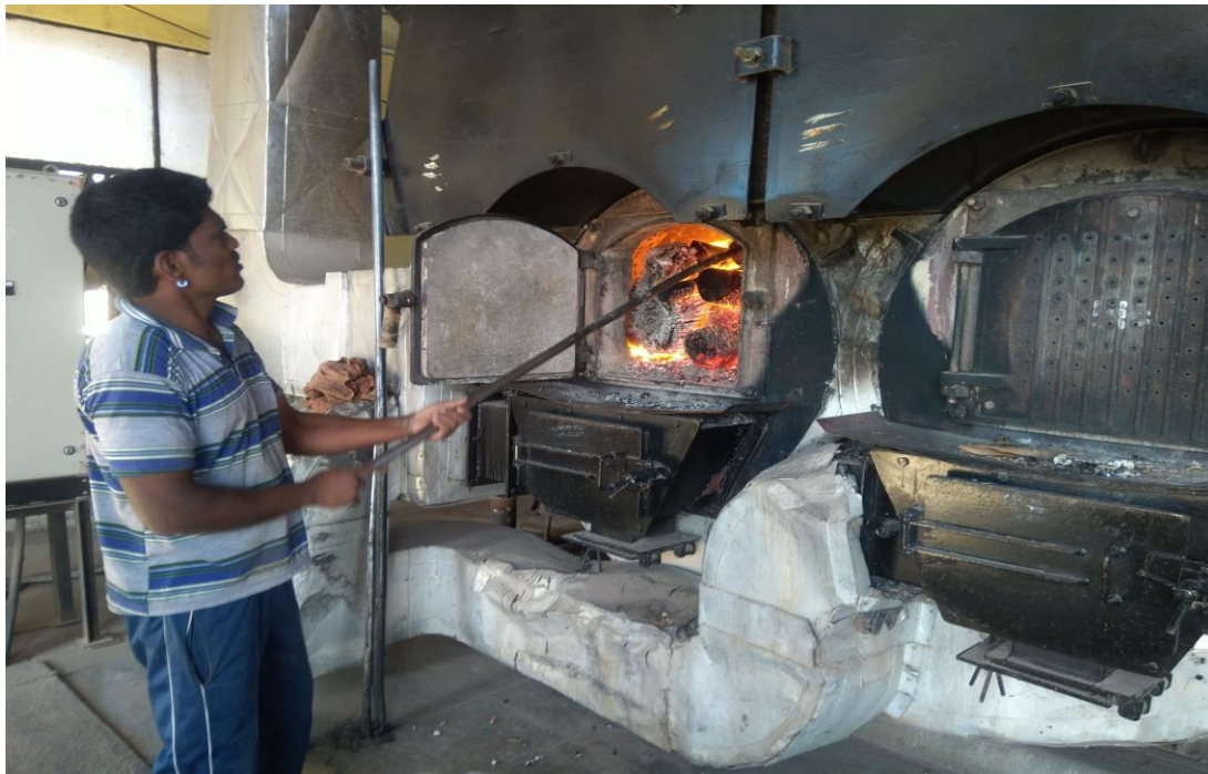
Fireman filling wood logs in to the boiler
