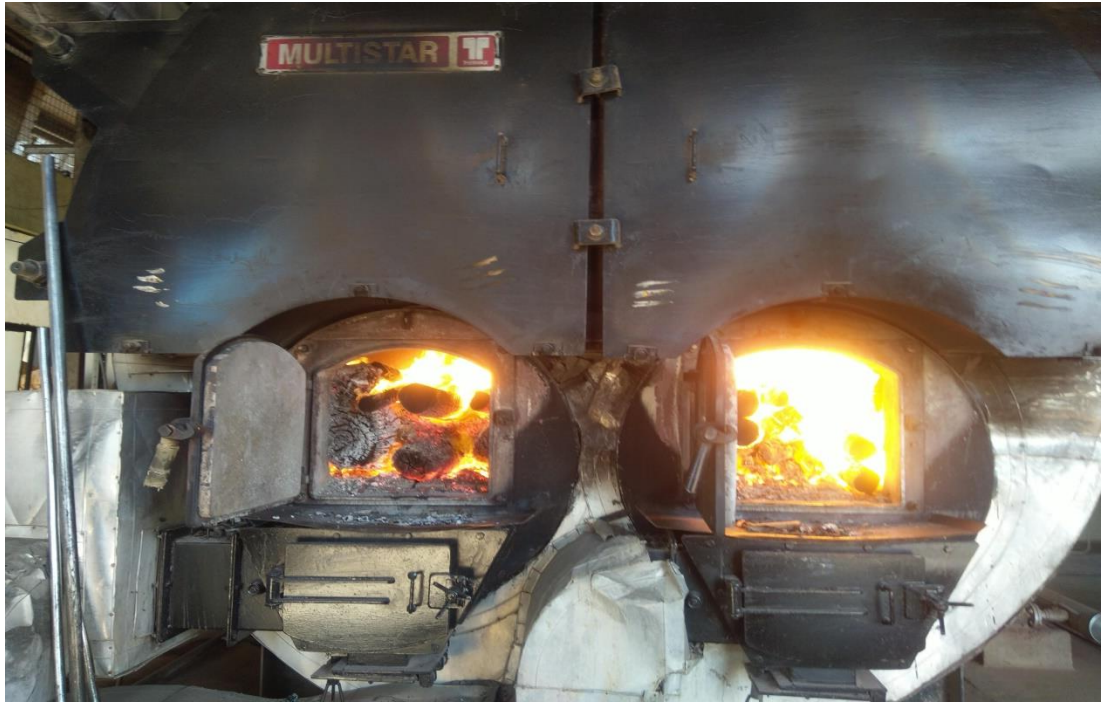
Fire wood boiler
