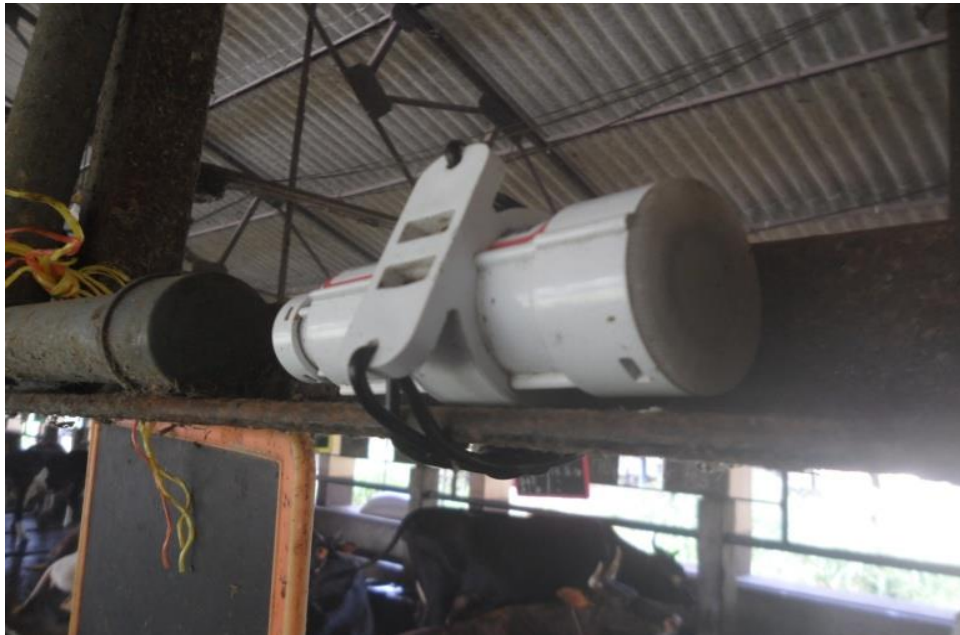
Plate 2.b. Hobo data logger installed in the animal shed
