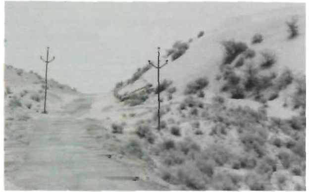
Road encroachment by sand
