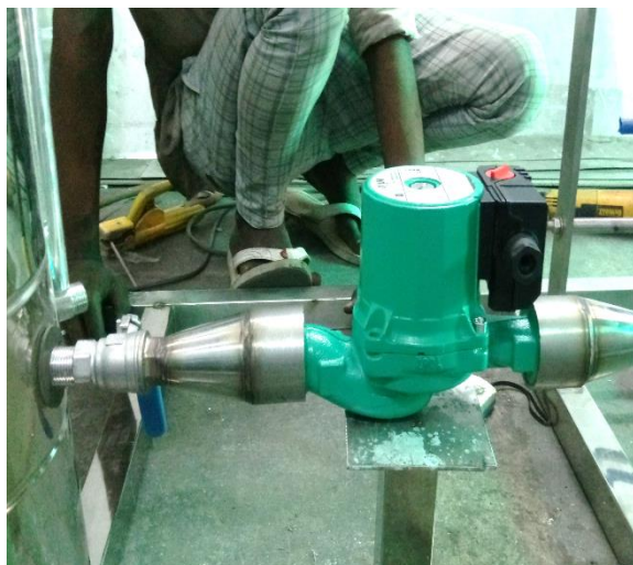
Hot water pump
