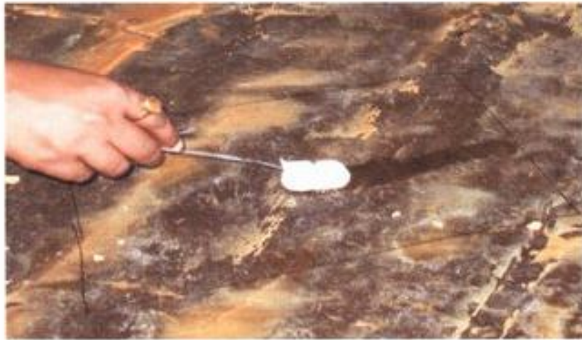
Plate 5. Swab Test of cooling pan
