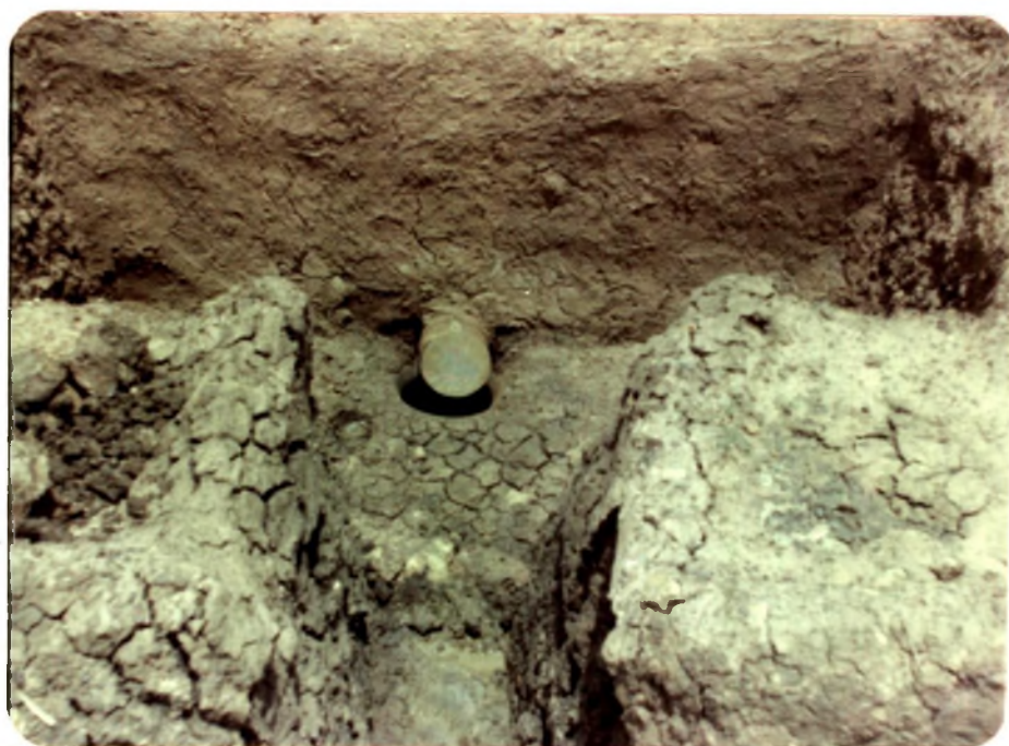
Plate 4. The outer end of tile drain protected with one way flap gate
