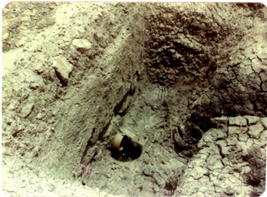
Plate 6. Plastic cisterns provided at the end of tile drains to measure tile drains out-flow.
