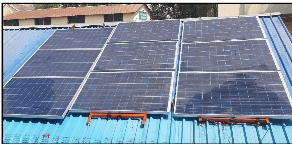
Plate 3.1 : Solar photovoltaic system for agro-processing unit
