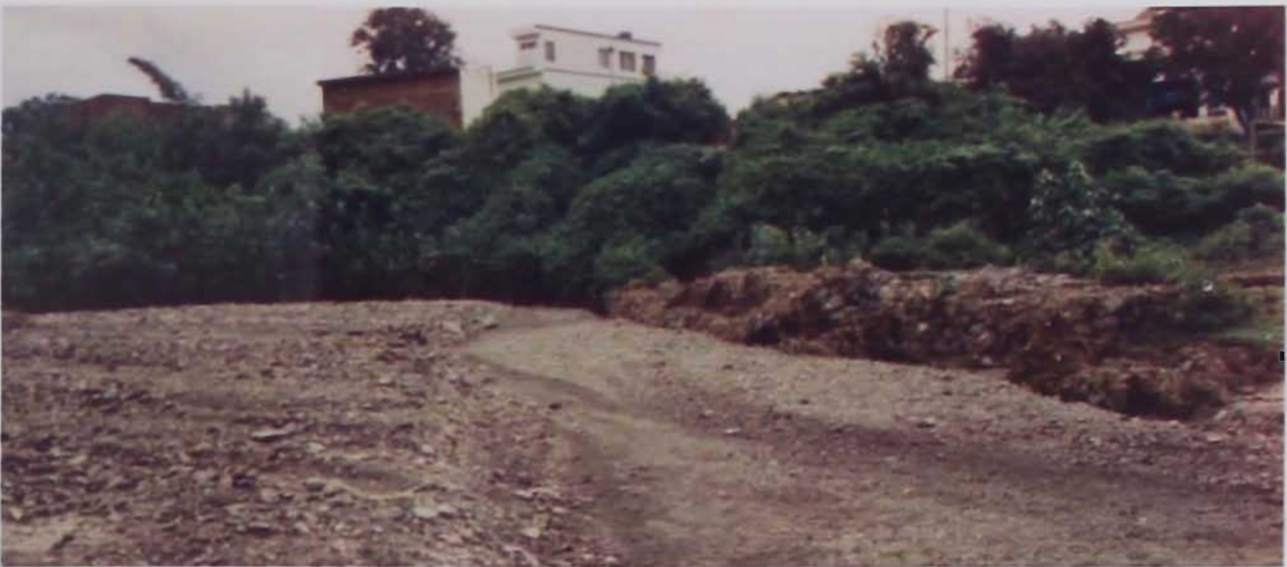
A. Damage to engineering measure (Spur)
