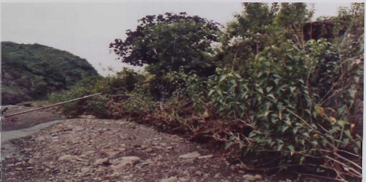
C. Damage to vegetative spur by flash flood
