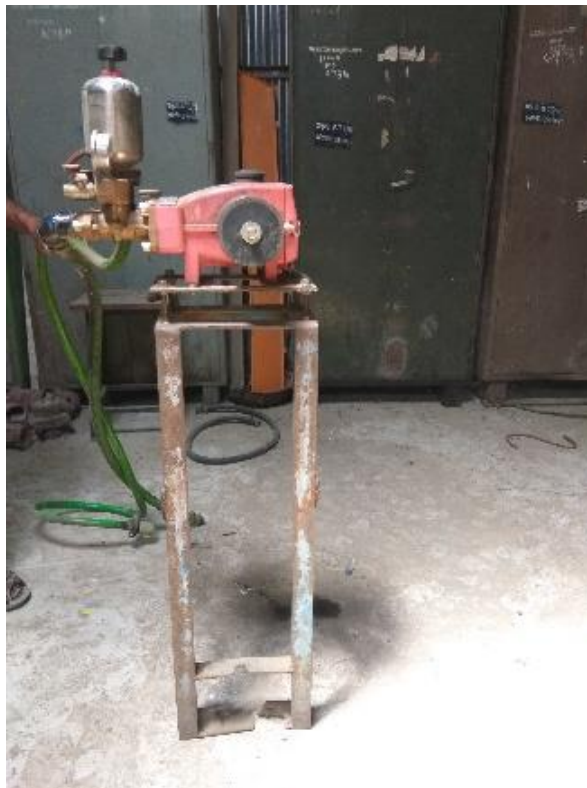
Fig. 3.3 Supporting frame of HTP pump
