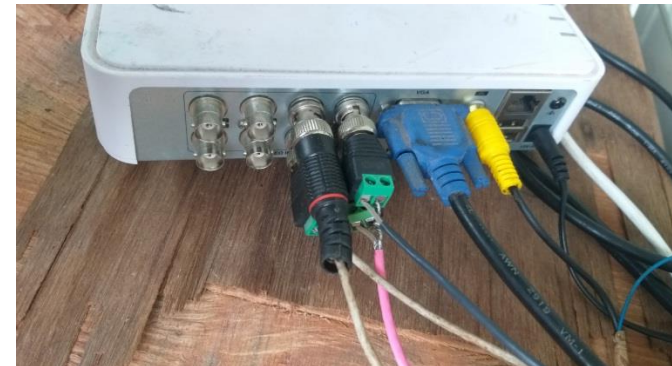
Plate No.3.4 : DVR machine fitted with CCTV camera cable
