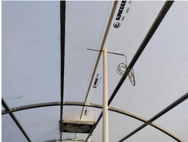
Plate 3.7 K-type sensors for temperature measurement
