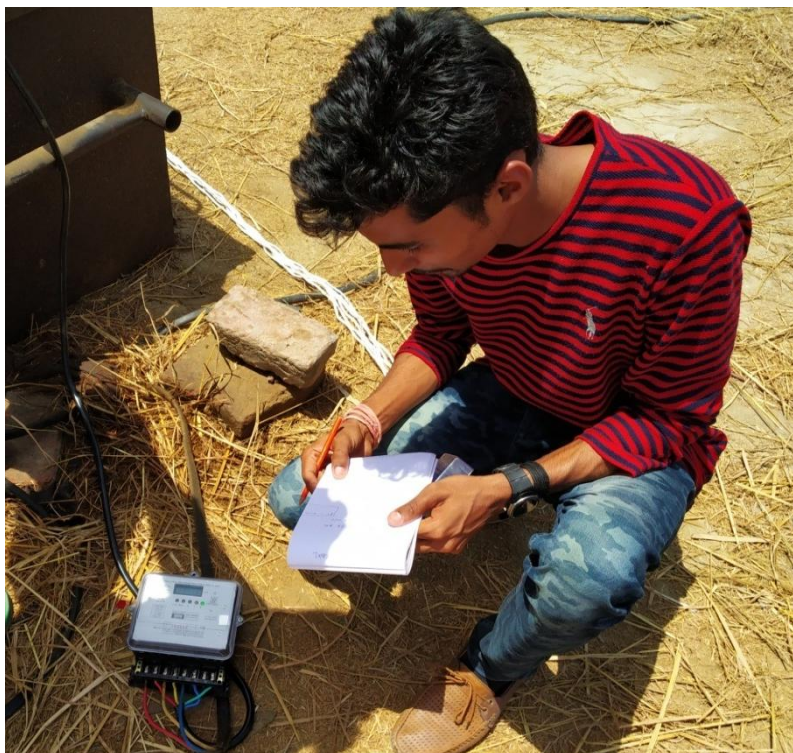
Plate 3.10 View of units consumed being recorded with energy meter
