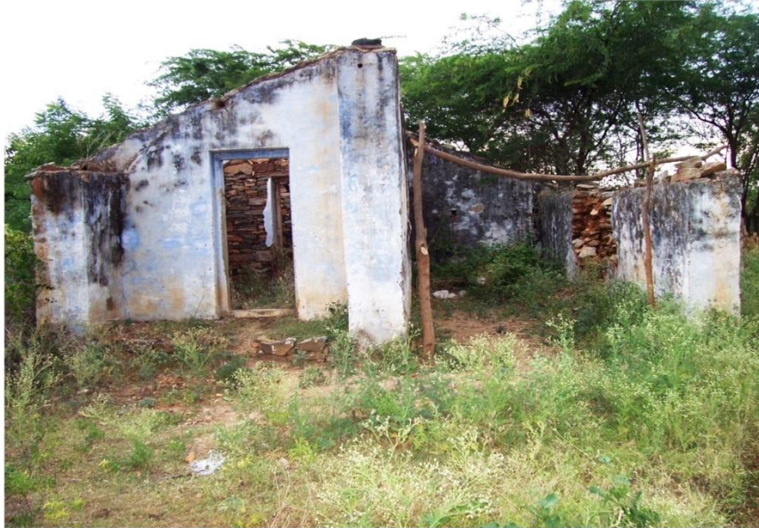
Plate 2. Dilapidated building housing feral colonies
