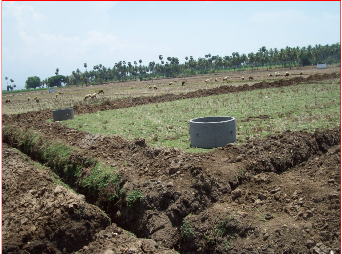
Plate 3.5 Trenches dug for laterals and collector with inspection chamber rings (Sumps) placed in the field.
