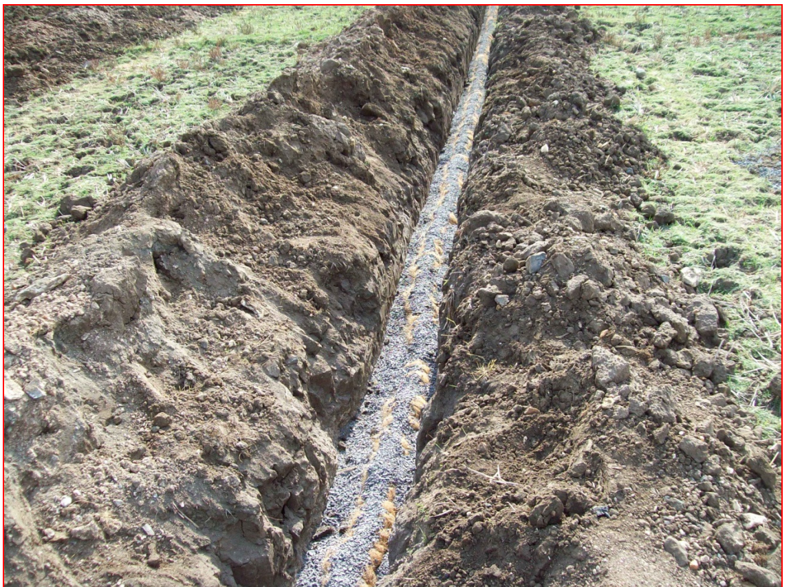
Plate 3.9 & 3.10 Placing 2.5 cm thick bedding material (zero chips) below and above the drain pipes (coconut coir enveloped)
