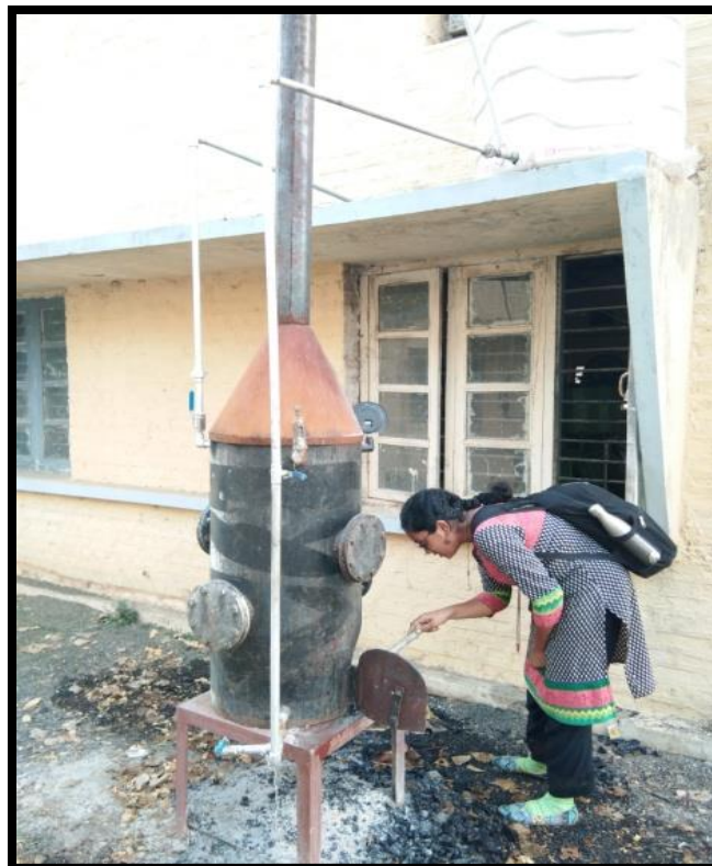
Plate 3.7 Feeding of wood as fuel to the boiler
