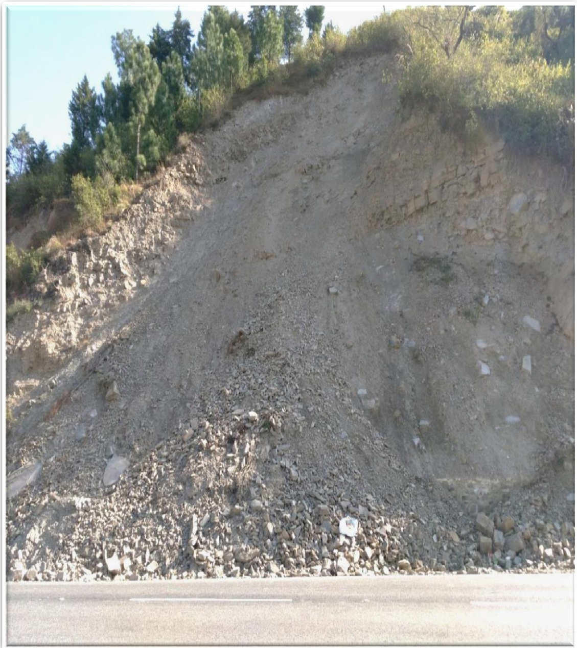
Fig. 3.4 Site View of Kakri Ghat NH 109 (after landslide 2018)
