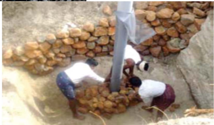
A pit around the existing bore well is filled with stone pellet filler material
