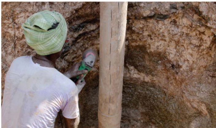
Small slot made on the casing pipe to allow rainwater to enter into borewell
