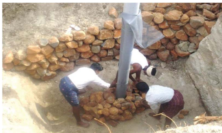
A pit around the existing bore well is filled with filter material
