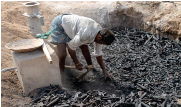
A pit around the existing bore well is filled with charcoal filler material
