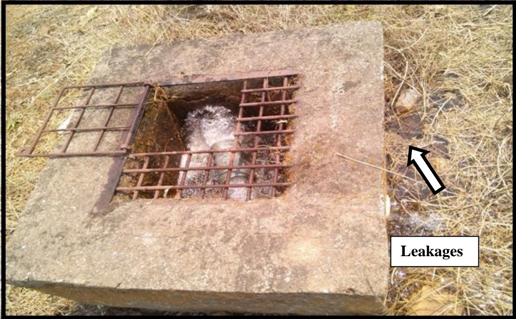
Fig 4.10 Leakages in hydrant
