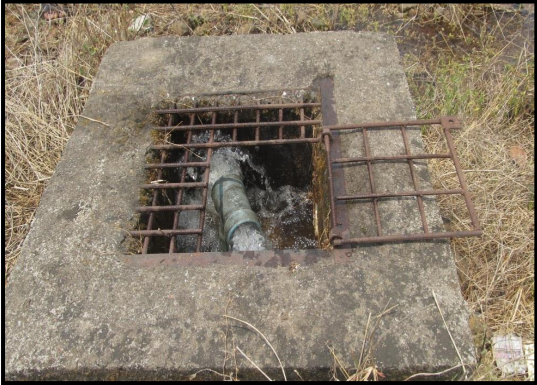
Fig. 4.9 Flow through hydrant (LBC outlet No.-1)
