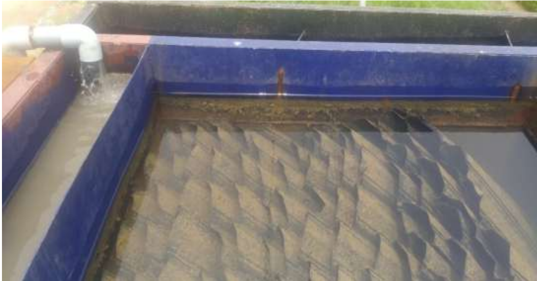
Fig. 4.10: Inclined tube clarifier while operation
