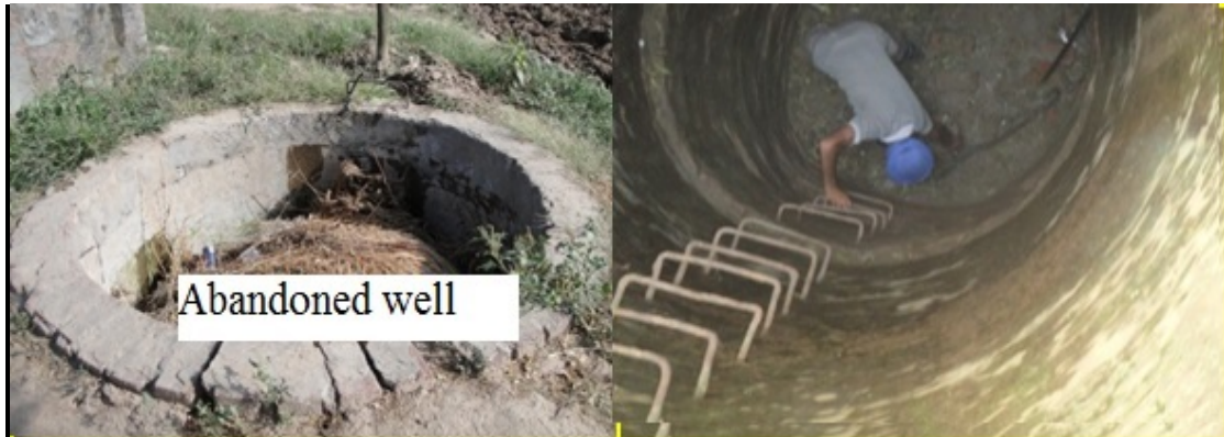
Fig. 3.3 View of uncleaned abandoned well at site 1
