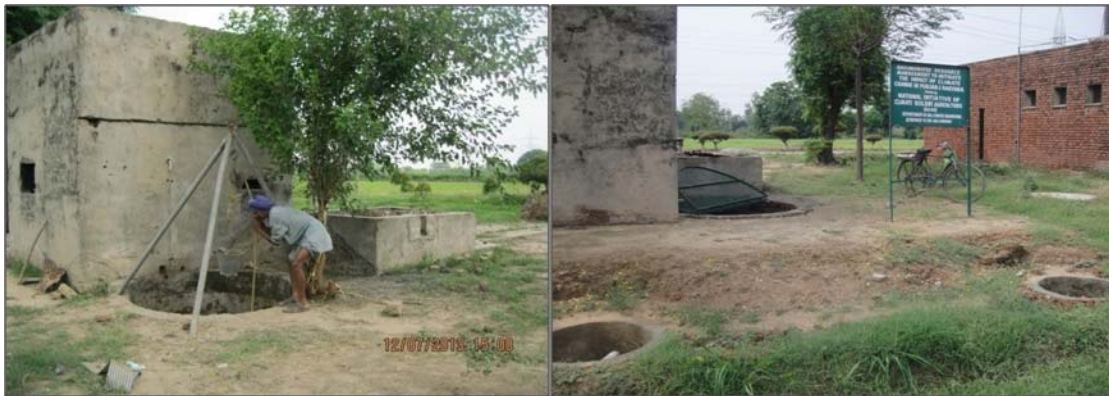
Fig. 3.4 View of uncleaned abandoned well at site 2
