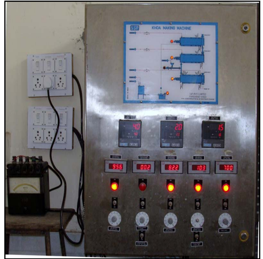
PLATE 3.1.1.6.9 c: Wattmeter with Switch Board in working condition
