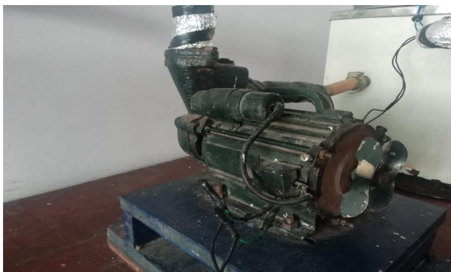
Fig 3.23 Picture of water circulating pump
