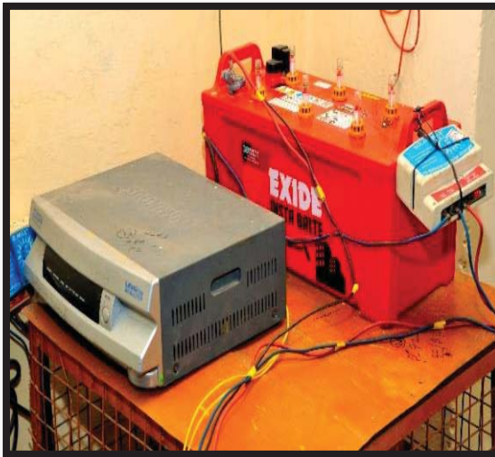
(g) Inverter, battery and MPPT
