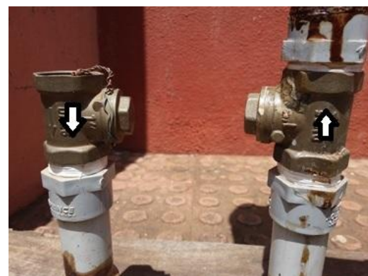
Plate 3.35 Alignment of Non-return valves
