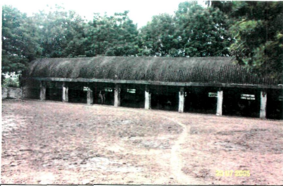
Plate I Cow shed at IF showing (a) canopy of trees (b) Dome type roof
