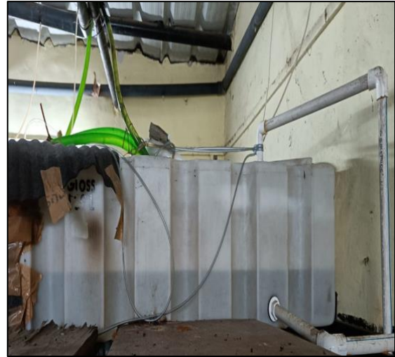
Plate 3: Overhead storage tank
